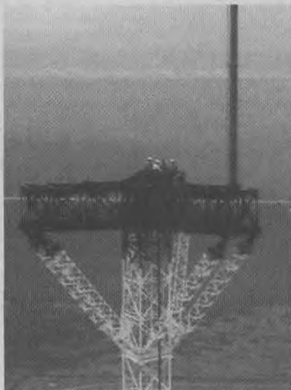
HC Jefferies Tower crew attaches the base plates for two new antennas in January 2002. Attaching the base plates and antennas was accomplished in 3.5 hours.
